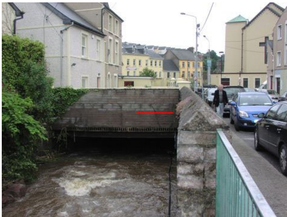
View of entrance to Orchard Court cuvlert after flood level reduced. Red line indicates level described as observed earlier. Based on Lee CFRAMS (7BRI_93) survey drawing this approximates to a level of about 9.4m OD Malin, and it is about 1.1m higher than the soffit level of the culvert entrance.
