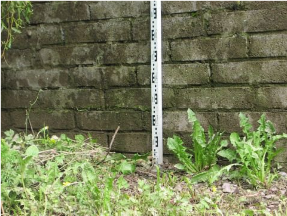
Photo showing tide line at about 0.27m on staff on inside of wall at exit from hotel grounds near north end of flood extent
