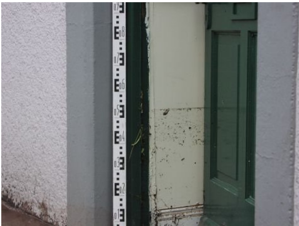
View showing depth of flooding in a house in Thomas Davis Street, (just over 0.5m).
